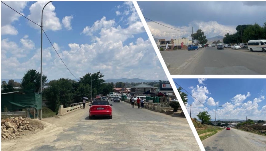
Figure 1: Roads Infrastructure is in a poor condition (roadworks are underway in some areas)
