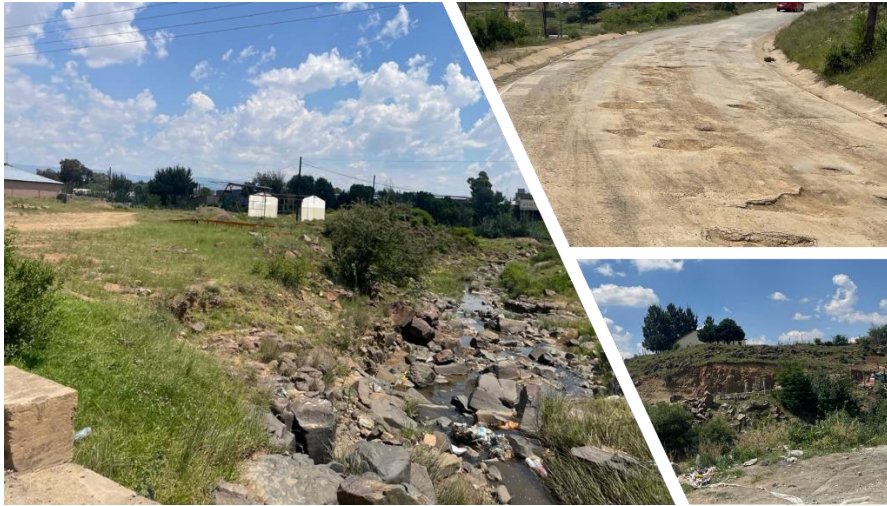
Figure 6: Degraded and Poor Stormwater and Management Evident
